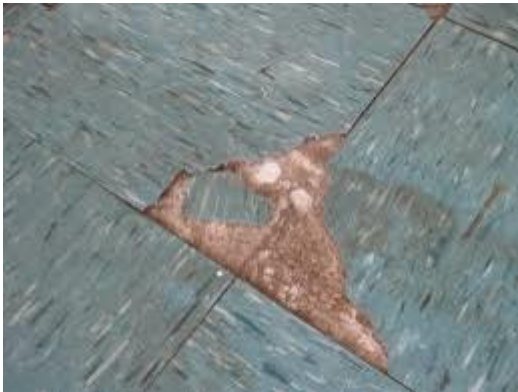
Asbestos floor tiles
